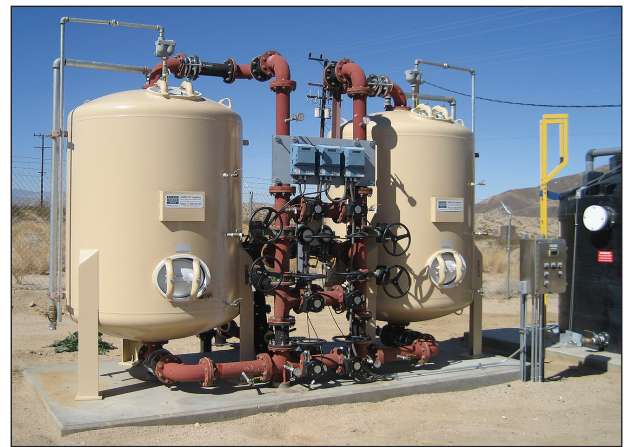
The arsenic removal system consists of two 5-ft-diameter adsorption vessels in parallel, tanks A and B, each containing 69 ft 3 of granular ferric oxide pelletized media.
