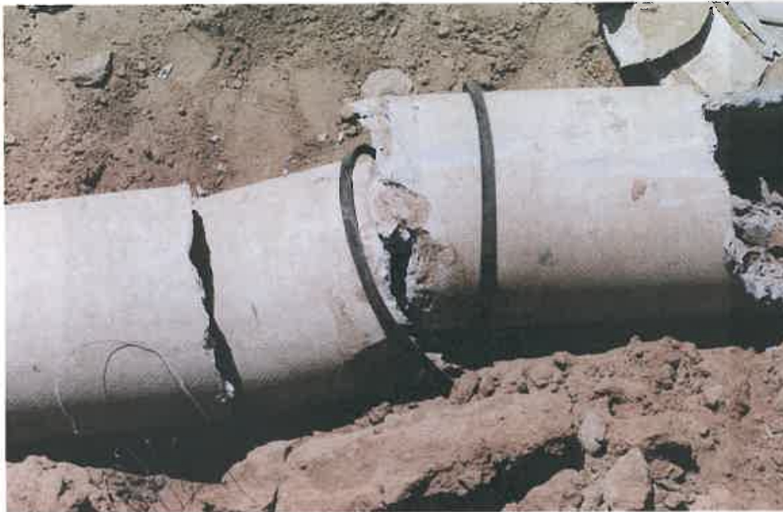
Earthquake, Ground Fracture and Pipeline Failure
