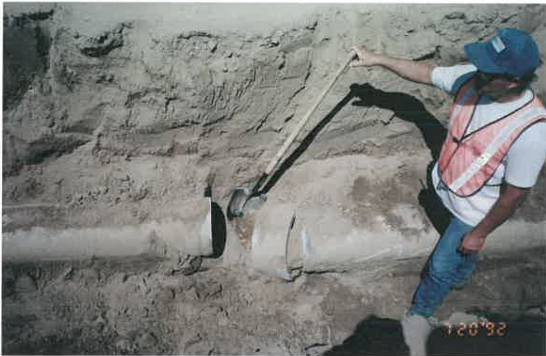
Earthquake, Ground Fracture and Pipeline Failure Above and Below
